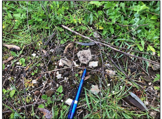
Asbestos cement sheeting fragments
